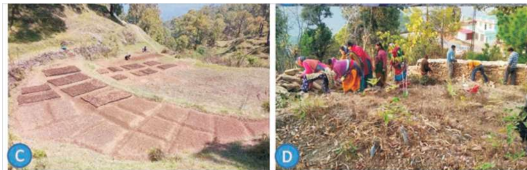
Figure 2: C) Land preparation for nursery development, D) Construction of protection walls through collective gender efforts
